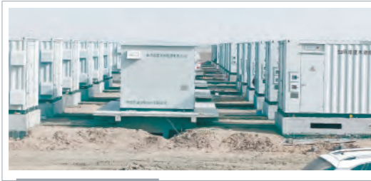
中石油塔里木油田伽师县600MWh光伏发电项目 CNPC's Tarim Oilfield 600MWh Photovoltaic Power Generation Project
