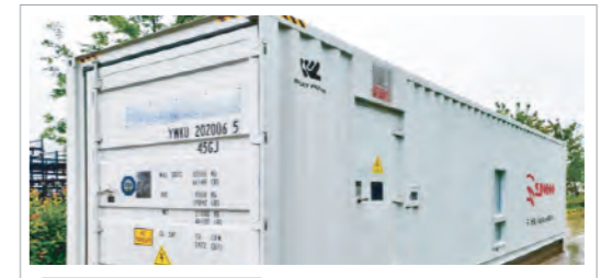
克罗地亚17MWh光储互补项目 Croatia 17MWh Photovoltaic and Storage Complementary Project
