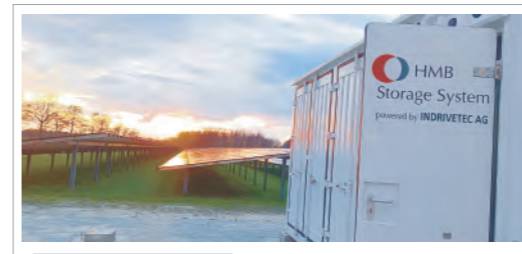
荷兰3.6MWh光储互补项目 The Netherlands Emmen 3.6MWh Photovoltaic and Storage Complementary Project
