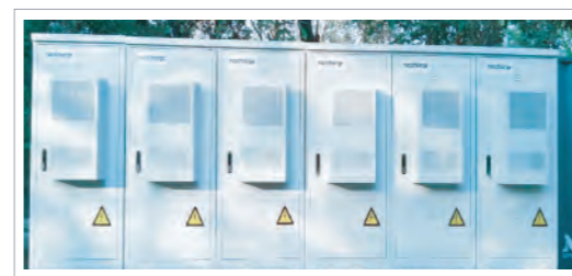
印度2MWh离网光储项目 India 2MWh High-Grid Photovoltaic Storage Project
