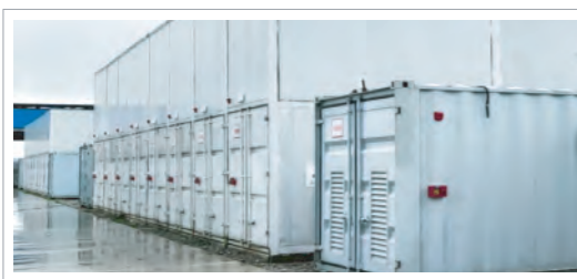
江苏央企造船厂100MWh 储能电站项目 State-Owned Shipyard 100MWh Energy Storage Station Project
